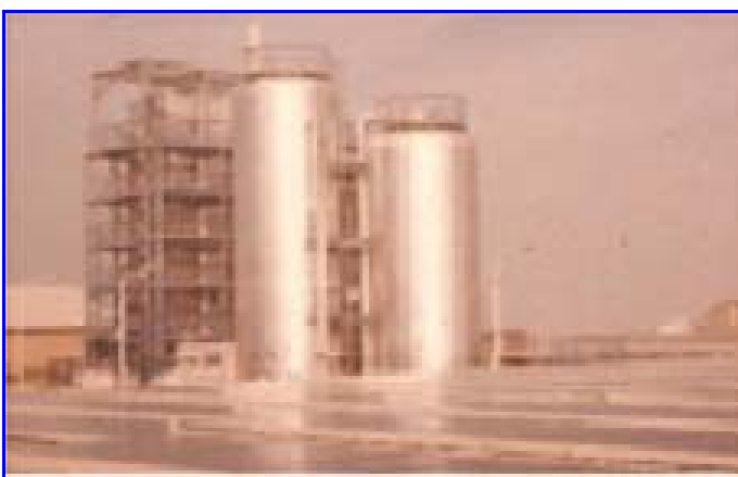
Fig. 7 Flat plate type solar collector and heated water storage tanks for MED desalination system (80m 3 /day) in Abu Dhabi, UAE
