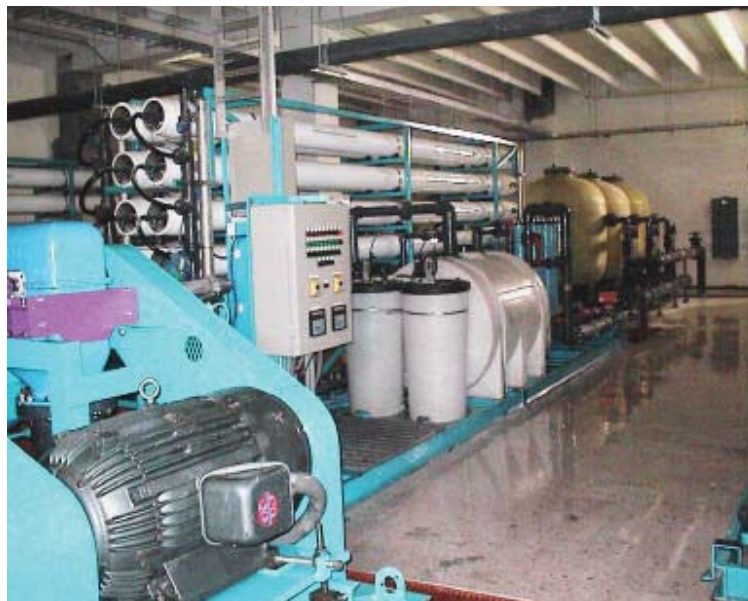
Fig. 2: An example of the Reverse Osmosis (RO) purification equipment used in the PS
