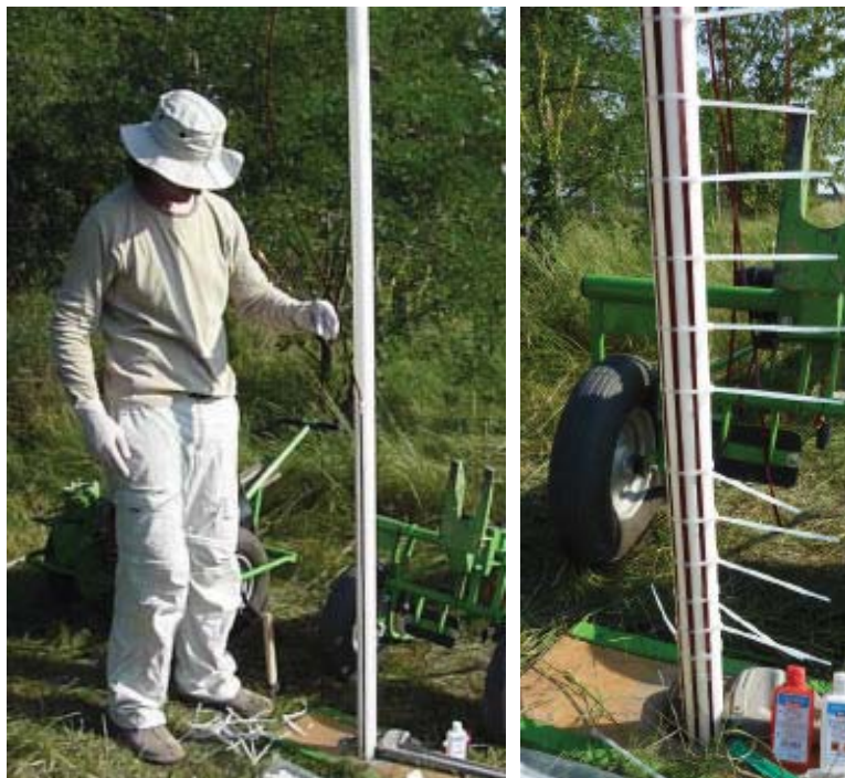
Fig. 2: Installation of the continuous TDR equipment into a predrilled boring at the August-Euler airfield
