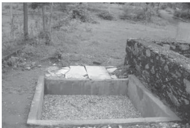
Fig. 2: Recharge of well through filtration pit
