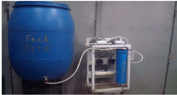
Fig. 2: Shows a photo of the entire membrane pre-treatment system
