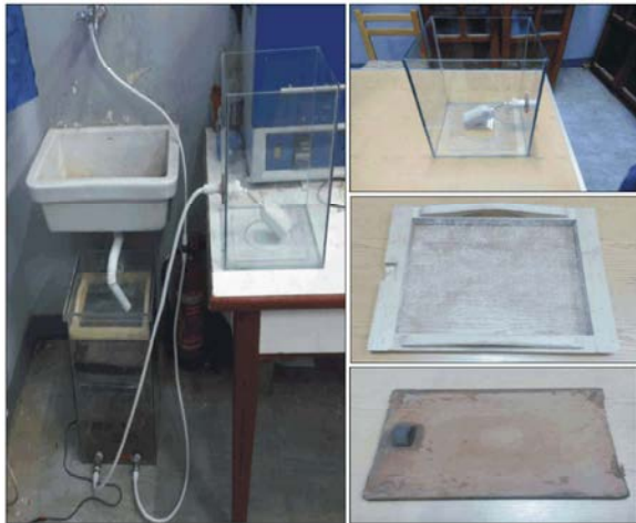
Fig. 6: A greywater treatment unit working by ceramic filters
